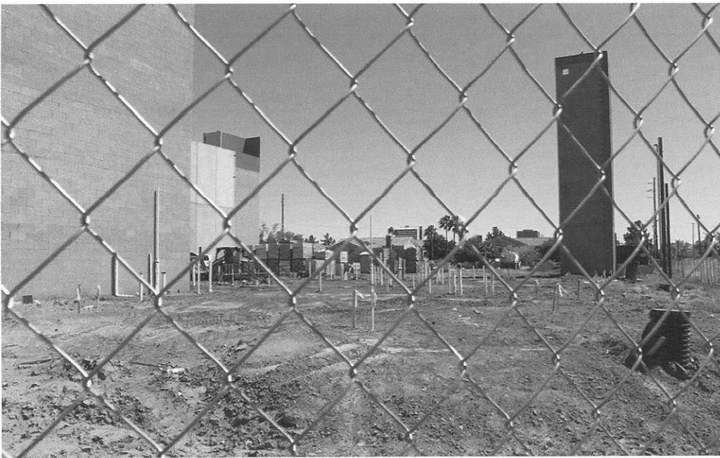
Construction is underway at the Aura Trinsic development site on Third Avenue and Coolidge Street, seen here on April 26, 2023. (Photo by Emma Peterson/Howard Center for Investigative Journalism)
