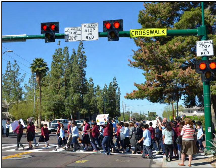
Pedestrian signal (HAWK) at the Phoenix Hebrew Academy at 515 E. Bethany Home Rd.
